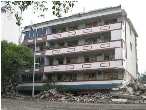
Figure 3. The overall collapse of the bottom layer
