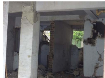
(a) Serious damage to the bottom seismic wall
