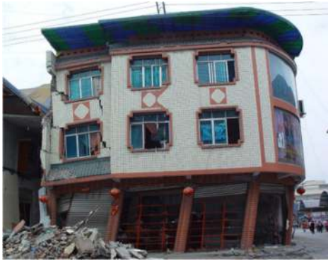
Figure 2. The bottom frame lateral displacement enlargement
