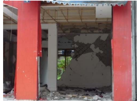
(b) Local collapse of the bottom seismic wall
