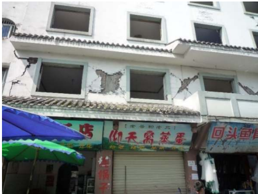
(a) Serious damage to a window wall
