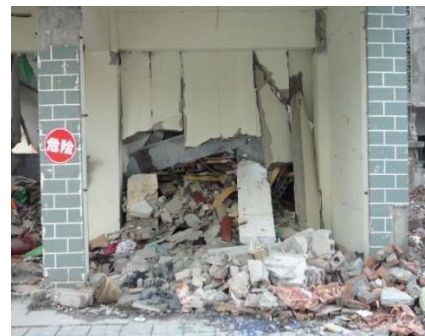
Figure 1. Serious collapse of a bottom frame story
