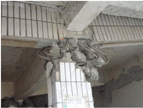
Figure 5. Serious damage to the top of a bottom frame column
