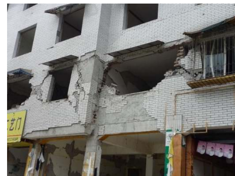
(a) Partial collapse of a transition layer wall
