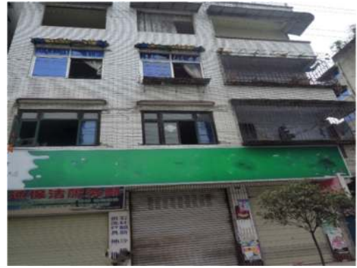
(a) The side of the mixed bottom frame structure near the street is basically intact
