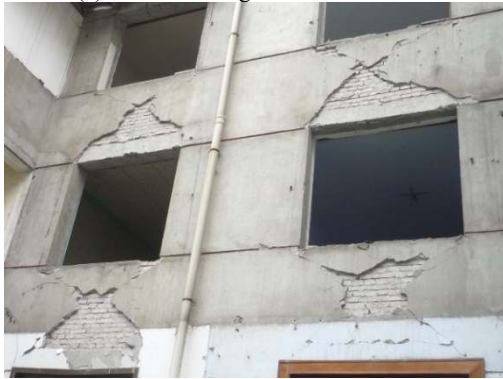
(b) Serious damage to the wall under the window
