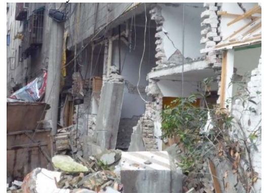
(b) Serious shear failure of the rear longitudinal wall on the side of the back street of the mixed bottom frame structure
