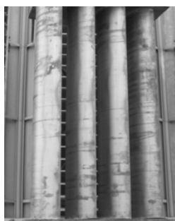
Figure 2. The guide vanes cascade installed in the cooling tower at Montazer Ghaem Power Plant
