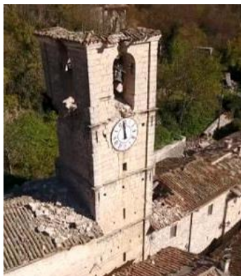
Figure 7. Belltower in Castelsant'agelo, damaged by the earthquake in 2016 (confined tower)
