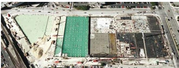
Figure 6. Construction site with steel sheet piles used as permanent and temporary retaining elements
