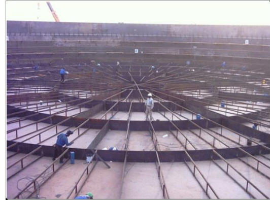
Figure 1. Lower deck and floating roof stiffeners configuration (courtesy of Kavan Sadid Sanaat Koosha)
