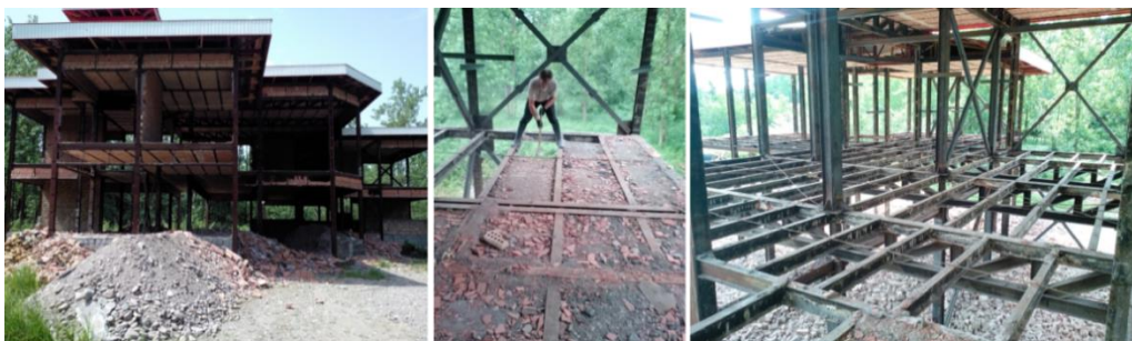
Figure 2. Demolition of the brick arch panel in a steel building to strengthen in Iran
