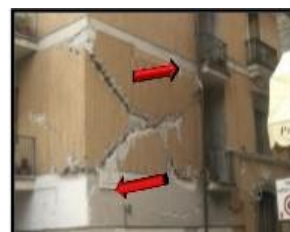
Figure 1. Diagonal cracking of infill
