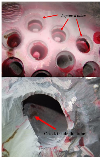
Figure 4. Damages of the tubesheet after five years of service
