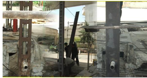
Figure 11. Photo of strengthening construction of a gas station in city of Tehran
