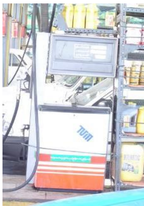
Figure 5. A typical pump used in gas stations in Tehran
