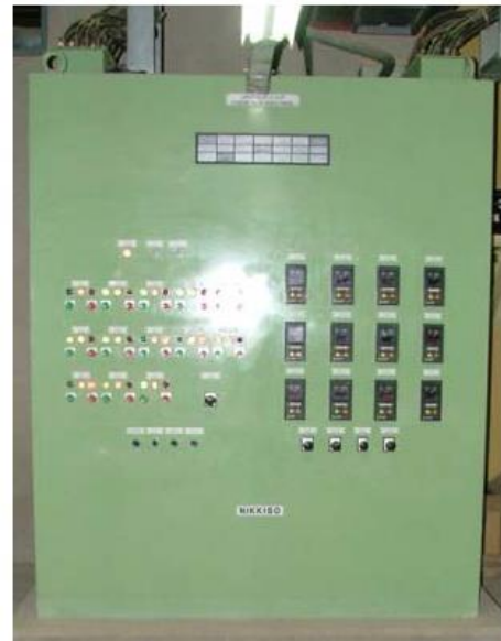
Figure 8. A sample of electrical equipments at the ground floor
