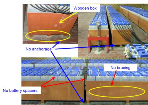
Figure 11. Some samples of battery racks with no anchorage, no bracing and no battery spacers concerns
