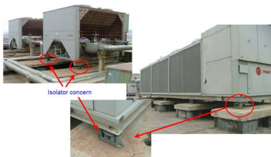
Figure 13. Some samples of equipments on the roof level which have rigid attachment and isolator concerns
