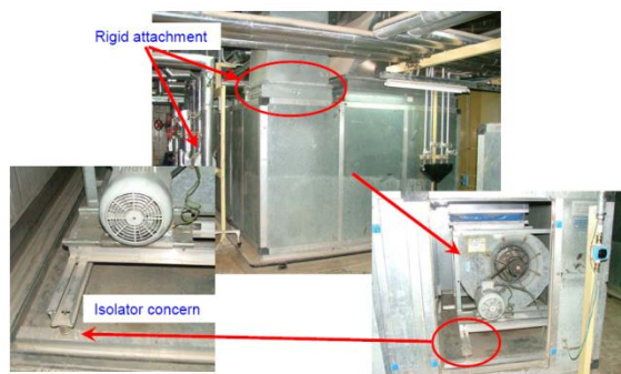
Figure 12. A sample of air conditioning equipments at the end story which has rigid attachment and isolator concerns
