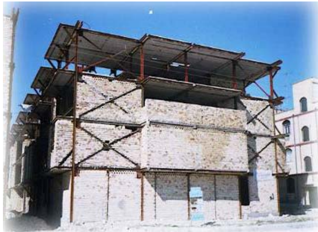
Figure 7. Soft story due to elimination of bracing in first story.
