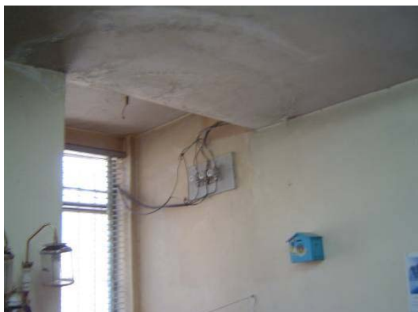
Figure 5. Effect of moisture on the building.
